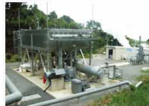
Binary-Cycle Geothermal Power Equipment
