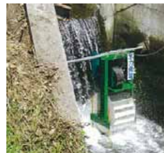
Hydropower equipment to generate 160W power utilizing a sewage treatment plant as a source.
