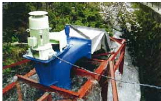
Panoramic view of the above hydropower equipment
